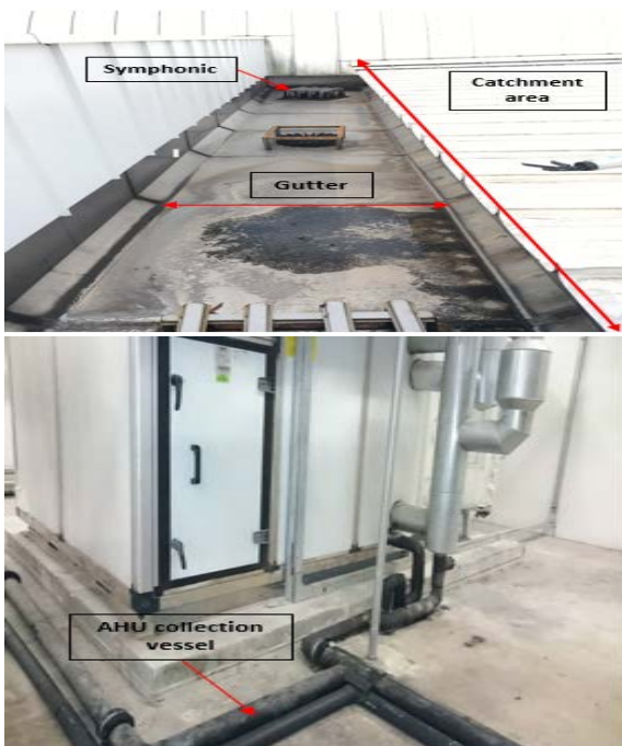
AHU Collection Vessel
