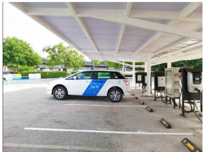
Charging station located at Suvarnabhumi Airport.
