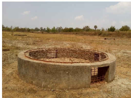
Ground water recharge wells at the recharge basin (R3)
