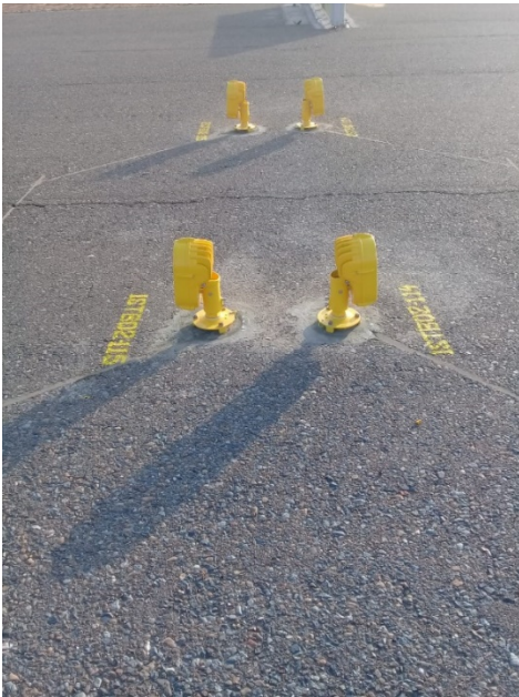
Elevated LED Stop Bar lights X 4
