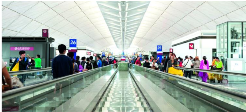
Caption 1 Lighting – LED Replacement Work in which 100,000 lighting were replaced with LEDs.
