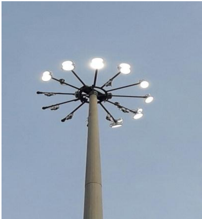
Caption 3 LED light fittings in Airside areas
