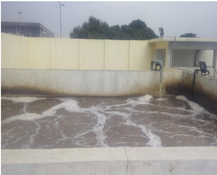
Caption 3 600KLD Sewage Treatment Plant
