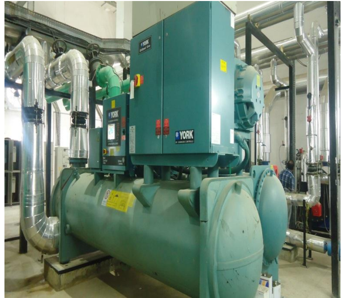
Caption 2 Energy Efficient Chillers
