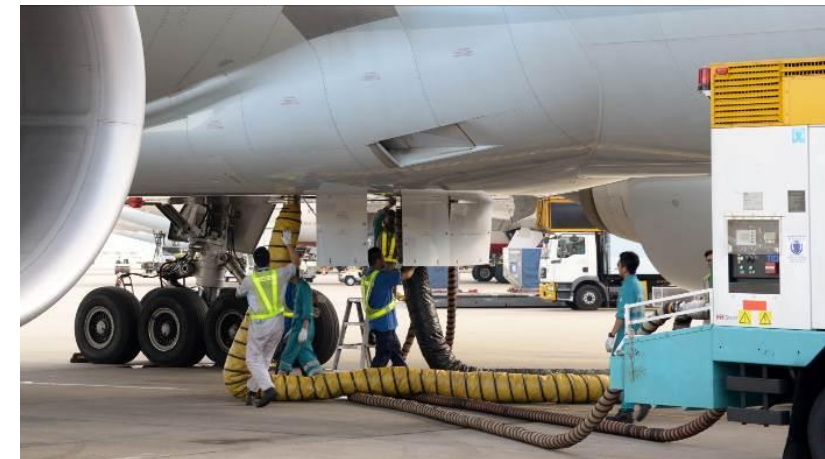
Caption 3 Apron Special System – Improvement Works for Fixed Ground Power (FGP) Units and Pre-conditioned Air (PCA) Units
