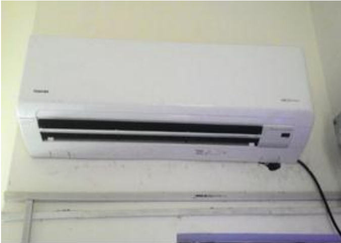
Caption 1 Energy efficient inverter A.C.s (inside view)
