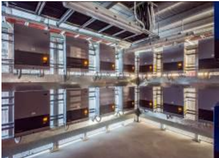
Caption 3 Inverter Room
