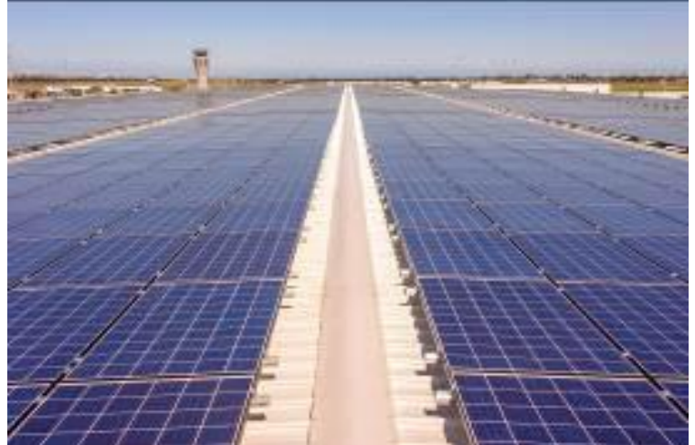
Caption 2 Rooftop View of Adelaide Airport Solar Installation
