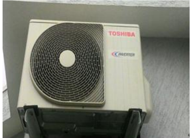
Caption 2 Energy efficient inverter A.C.s (outdoor view)
