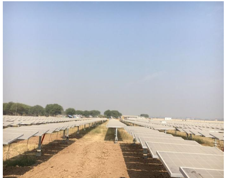
Caption 4 Grid Connected 3 MWp Solar power Plant
