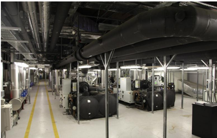
Caption 3 Heat Pump plant room
