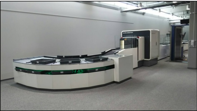
CT system installed at the screening checkpoint at CHUBU CENTRAIR International Airport
