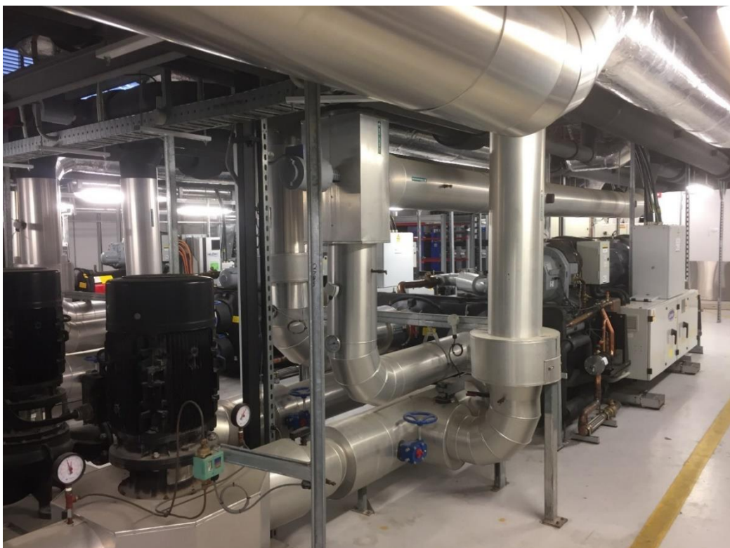
Ground source heat systems plant room
